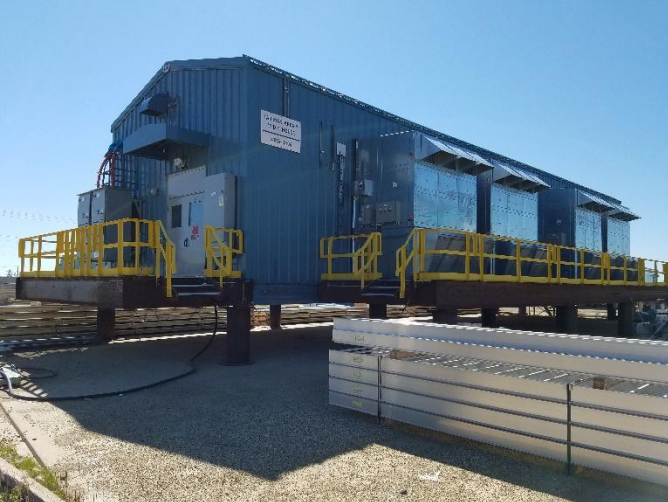
VFD Building for oil sands tailings
