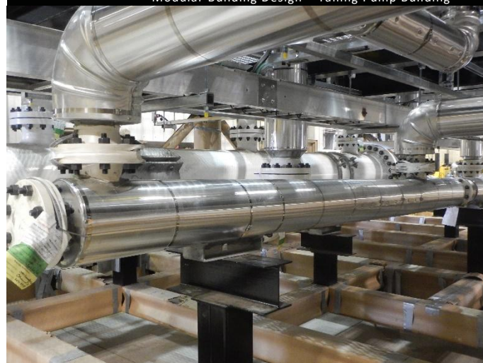
Metering Skid Including Heat Tracing
